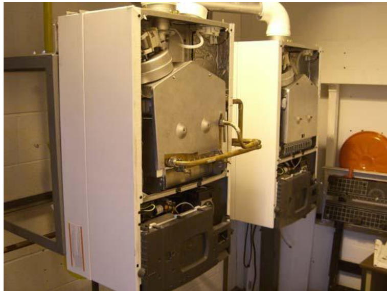
TPV Integrated Boiler System
